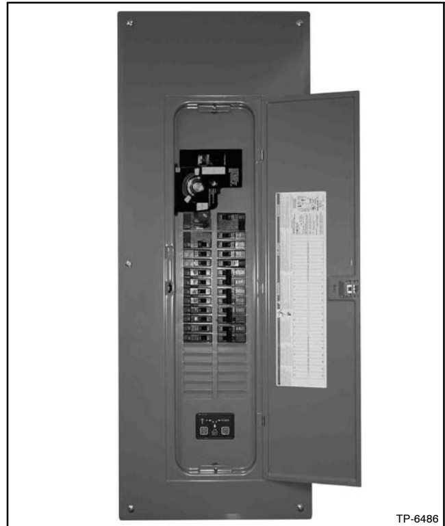
Figure 1 Intelligent Transfer Switch
