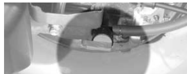
Fuel shutoff valve open.
