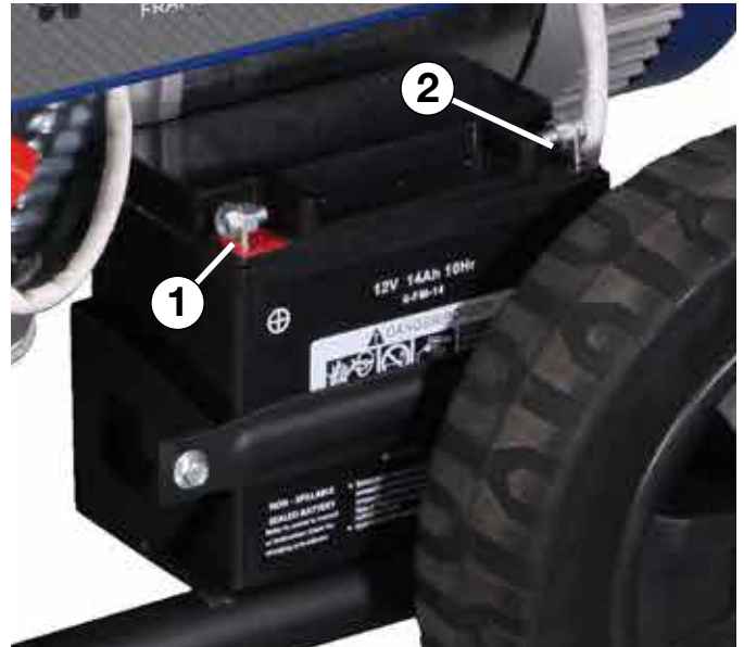
Attaching the Negative (-) Battery Wire
